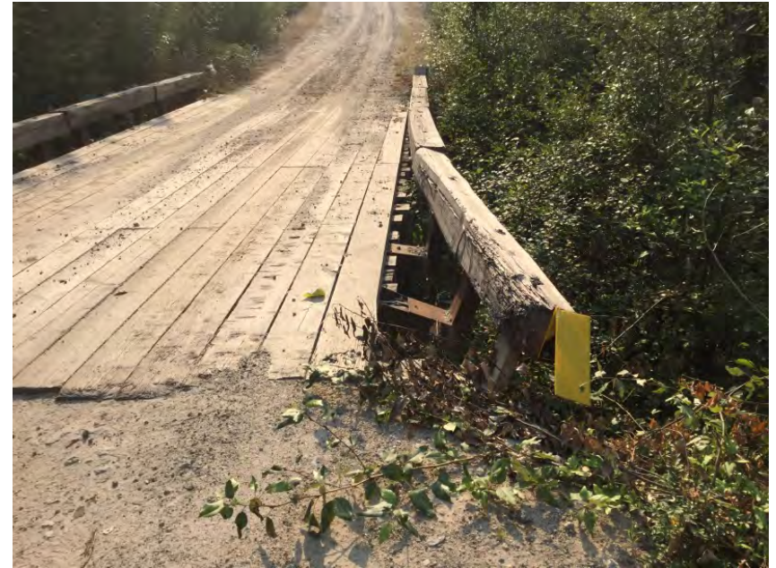
Damaged guardrail at downstream right approach
