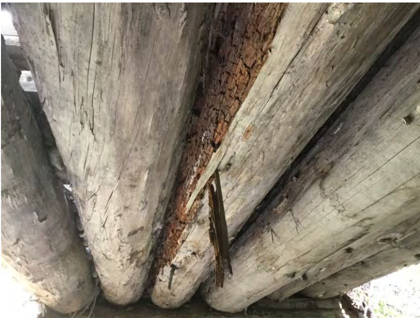
Log stringer condition
