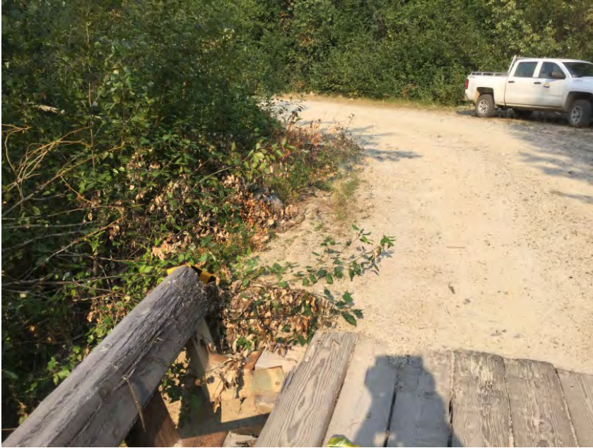
No fender log downstream right approach
