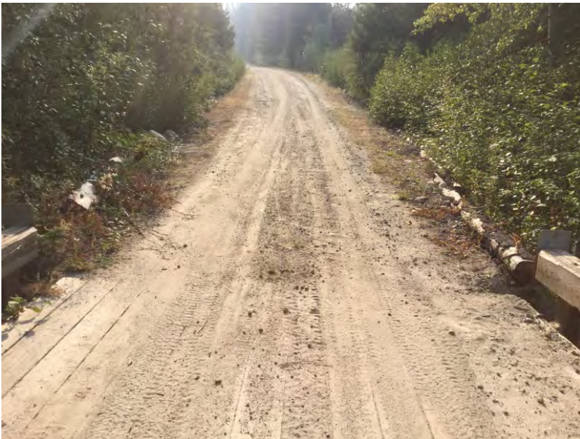
Insufficient log fenders at left approach
