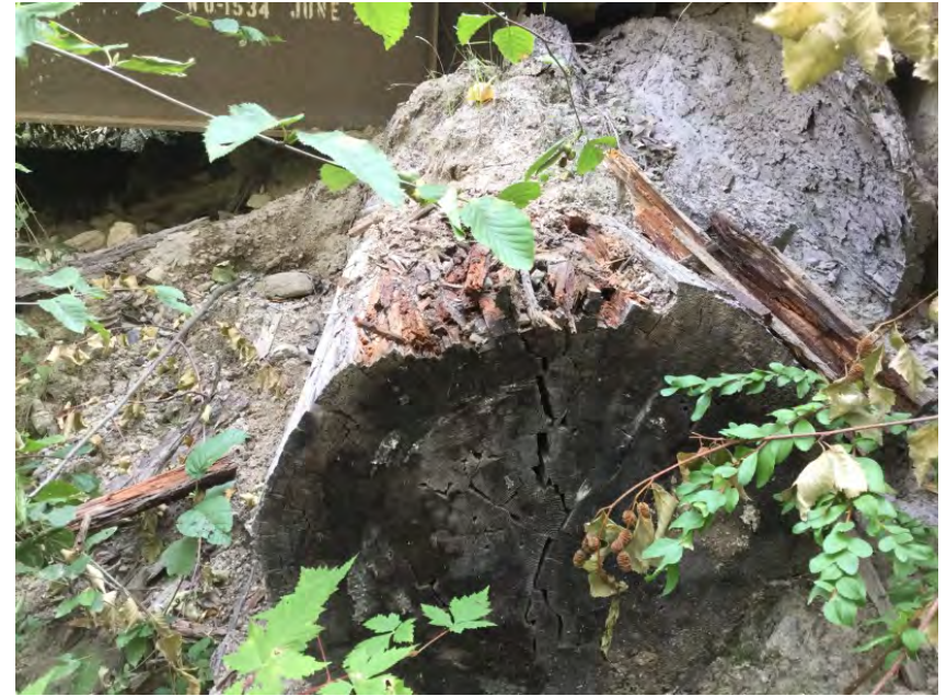
Log sill at left bank in poor condition
